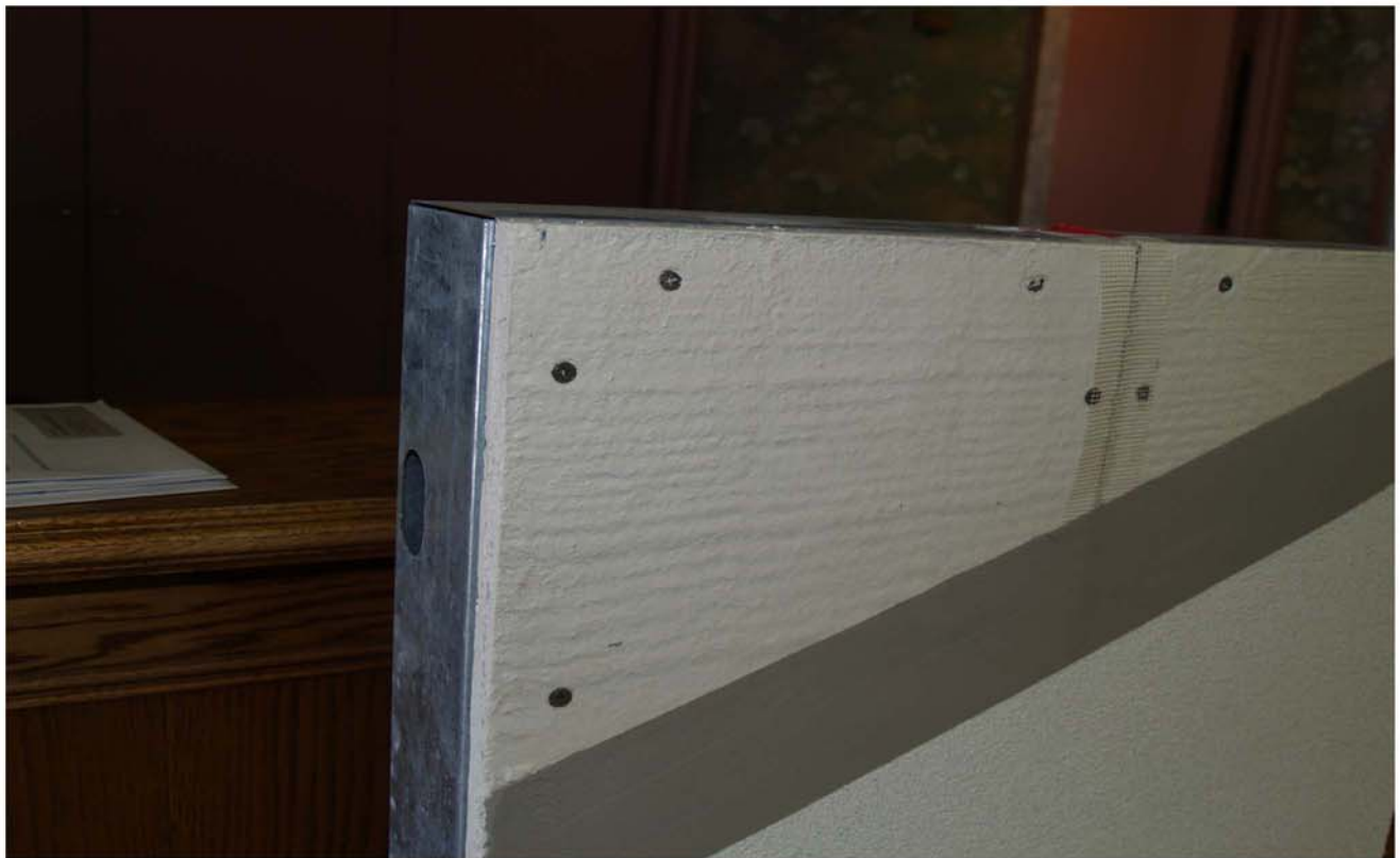
1 1/4 SELF - TAPPING DUROCK SCREWS W/ A 2" OR 4" TAPE ON SPLICES AND SEAMS, THIN LEVELING COMPOUND COAT AND 1 COAT OVER THE TOP
