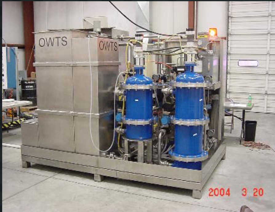
OWTS FILTRATION SYSTEM
